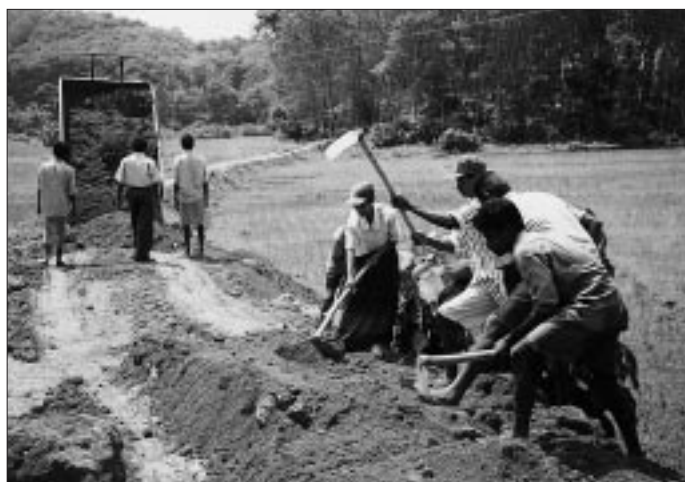
Building the road to Ratnapura, communities forging their own solutions, Sri Lanka
